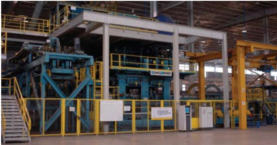
Fig 1. The new moulding machine at Technocast SA de CV, designed for a production rate of 90 moulds per hour
